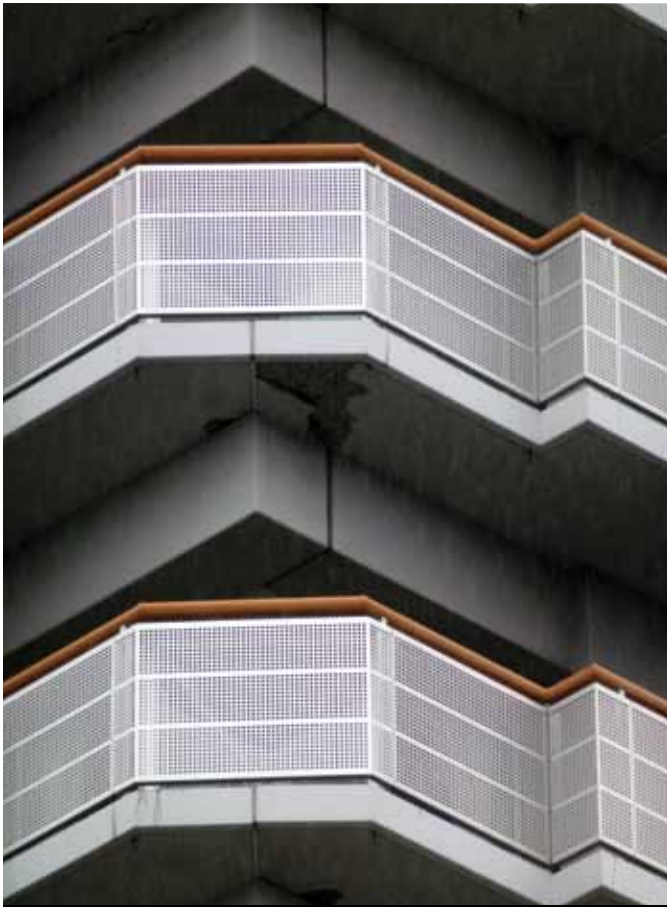
Figure 6. Spalling of slabs at corners of Namagachi Lions Tower.
