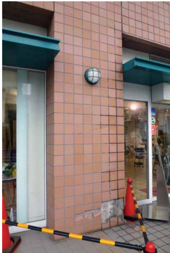
Figure 5. Minor spalling at the base of the columns of Namagachi Lions Tower.
